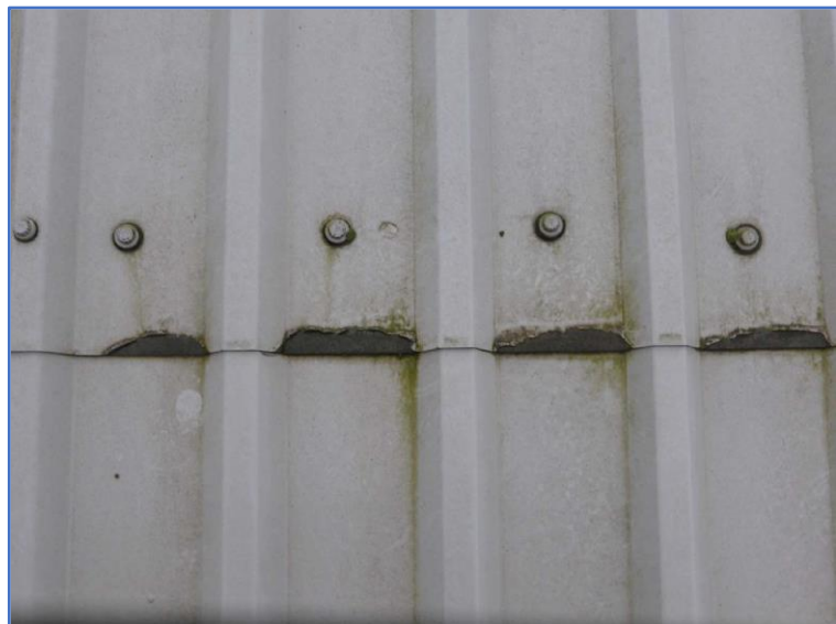
Figure 5.3 – Cut edge corrosion and premature breakdown of paint system at roof end lap detail
