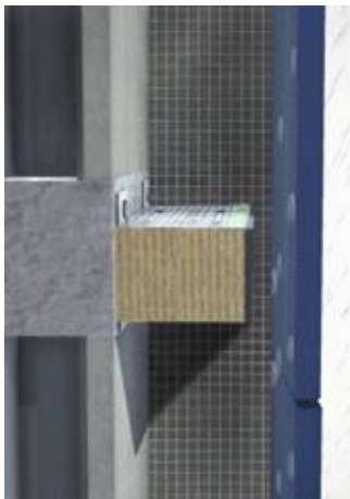
Horizontal open state cavity barrier installed so that the correct air gap is maintained to allow ventilation of the cavity
