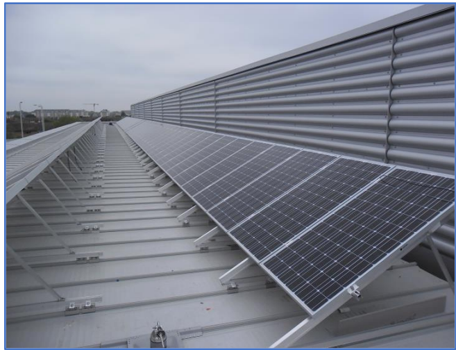
Figure 1.11 – PV panels installed on pitched frame connected to roof sheets
