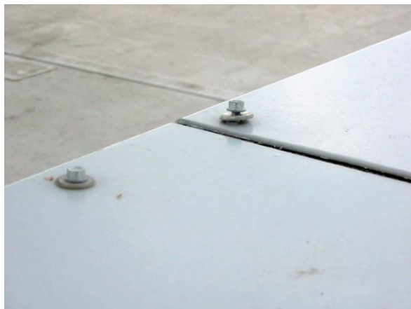
Figure 8: Consequence of no movement allowance at fastener location: fastener backing out of a capping
