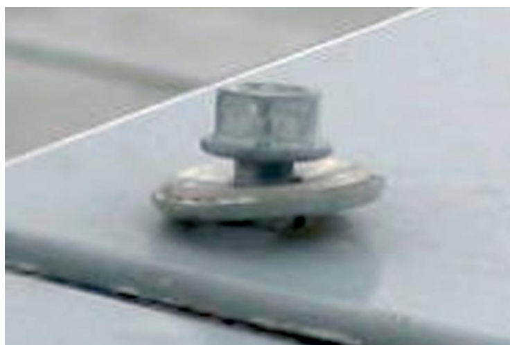
Figure 11: Fastener backing out of a capping: deformed washer indicates over-driven fastener
