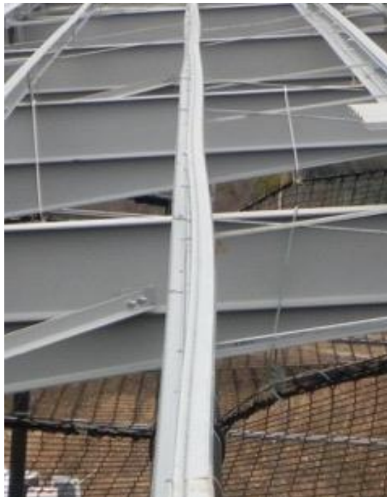
Excessive purlin rotation before any load applied
