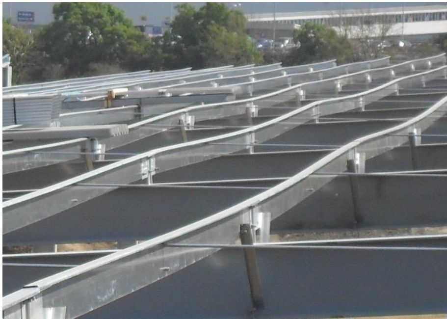
Primary steelwork installation tolerances affect secondary steelwork and then the roof sheeting unless corrected
