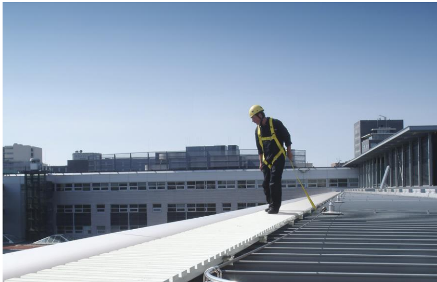
A typical cable system and walkway
