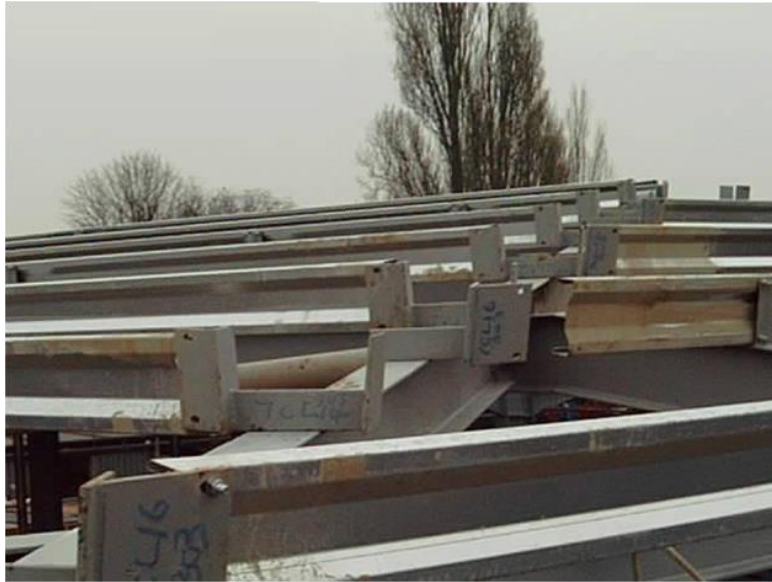
Image 3: Incomplete structural connections
