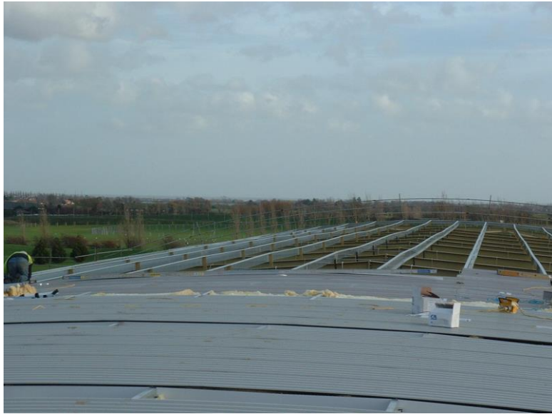
Image 1: Undulating/out of position purlin
