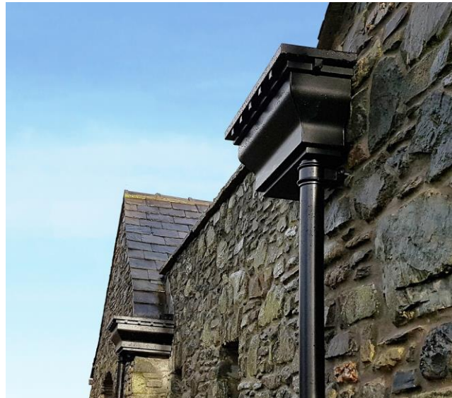
Hoppers and downpipe
