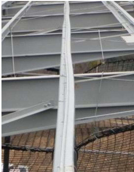
Excessive purlin rotation before any load applied
