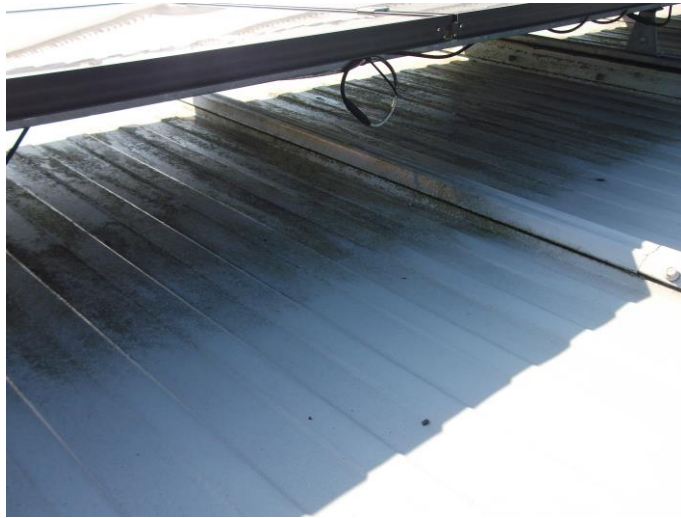
Area of cladding under a PV panel showing the build-up of dirt and algae
