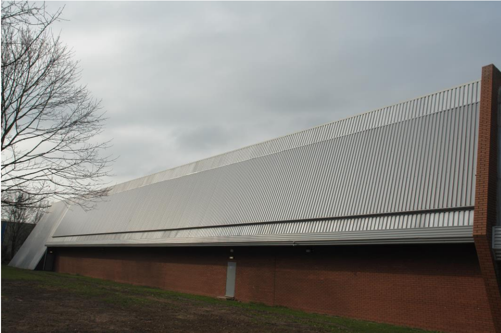
Solarwall used at Jaguar/Land Rover, Leamington Spa Image courtesy of C A Building Products
