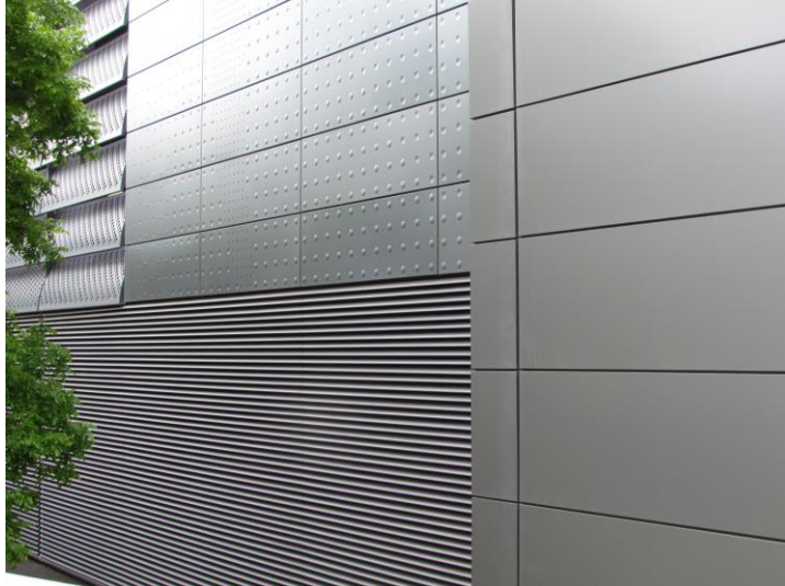
Just three of the profiles and panels integrated into the metal envelope
