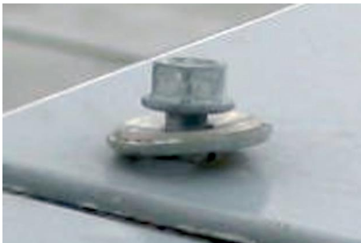
Figure 8: Consequence of no movement allowance: fastener backing out of a capping – deformed washer indicates heavily overdriven fastener
