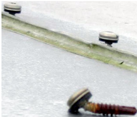
Figure 6: Consequence of no movement allowance: fastener shape demonstrates the high thermal movement loads developed. Carbon steel fastener corroding, stainless steel advised for flashings
