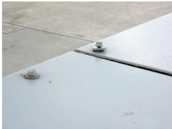
Figure 5: Consequence of no movement allowance: fastener backing out of a capping
