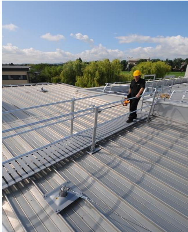
Collective fall protection of guardrail and walkway with accompanying cable system providing access to restricted areas
