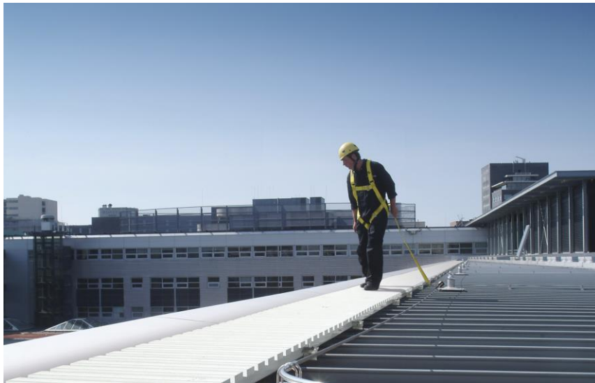
Collective fall protection of guardrail and walkway with accompanying cable system providing access to restricted areas
