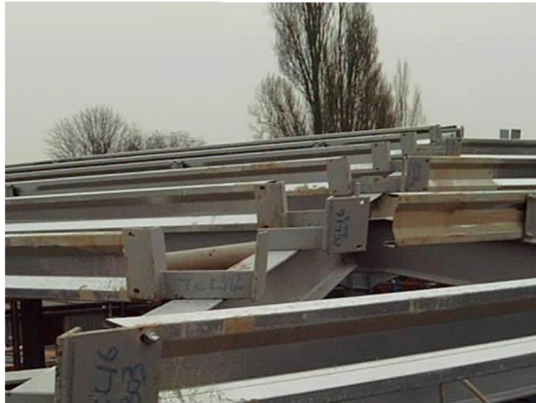
Image 3: Incomplete structural connections
