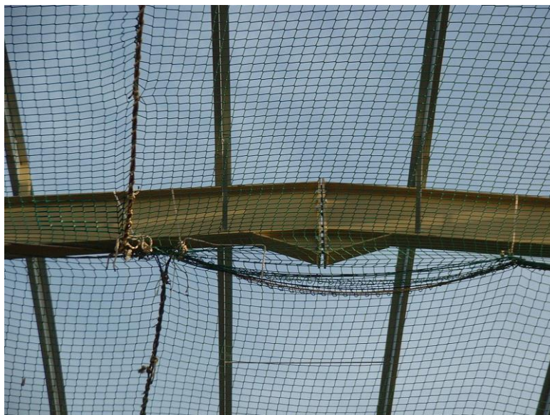
Image 2: Incomplete structural connections
