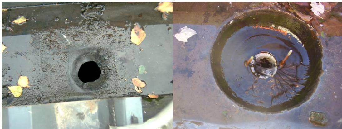
Fig 3 Gravity (left) and siphonic (right) outlets restricted by installed liners
