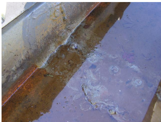
Fig 1 Metal gutter suffering corrosion and joint leakage
