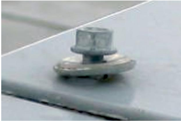
Figure 8: Consequence of no movement allowance: fastener backing out of a capping – deformed washer indicates heavily overdriven fastener
