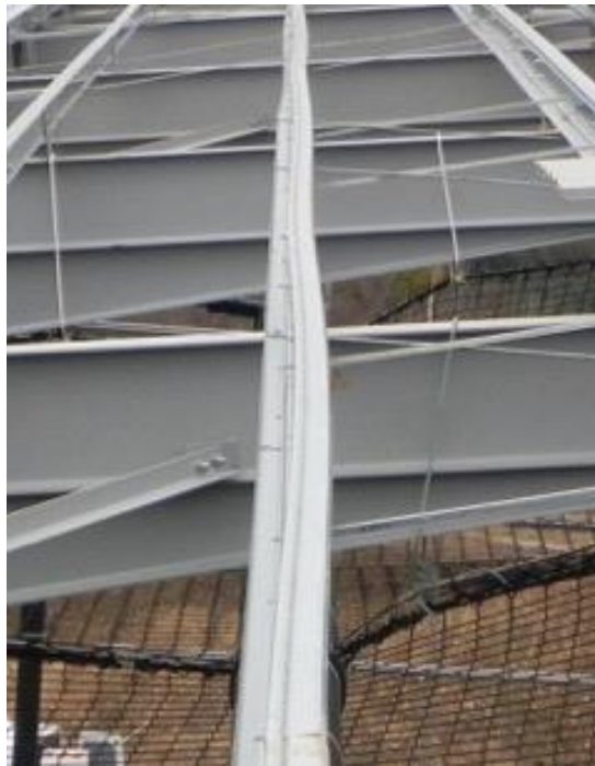
Excessive purlin rotation before any load applied
