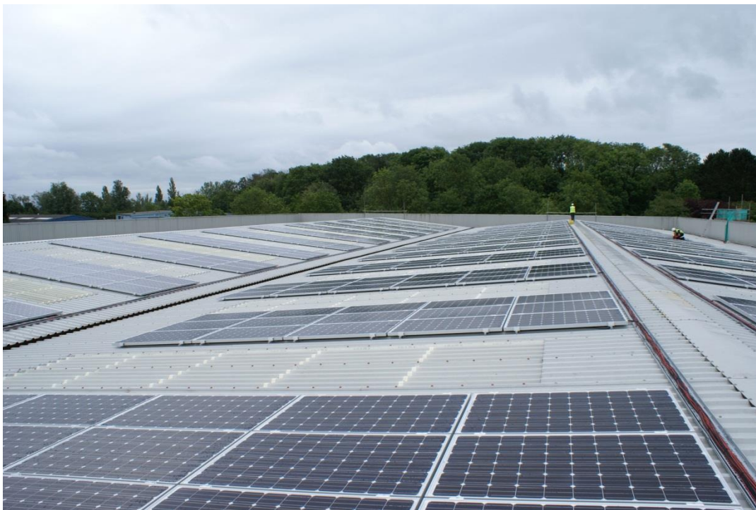
Solar panels fitted on the factory roof at Daventry
