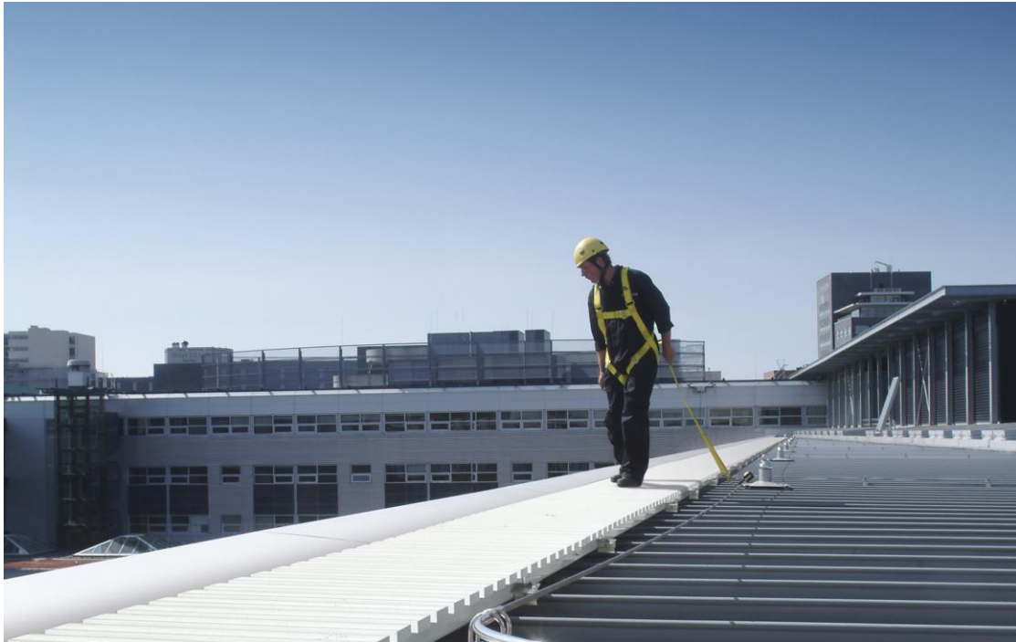
Collective fall protection of guardrail and walkway with accompanying cable system providing access to restricted areas. Image courtesy of Latchways plc
