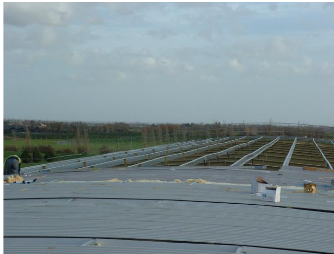
Image 1: Undulating/out of position purlin
