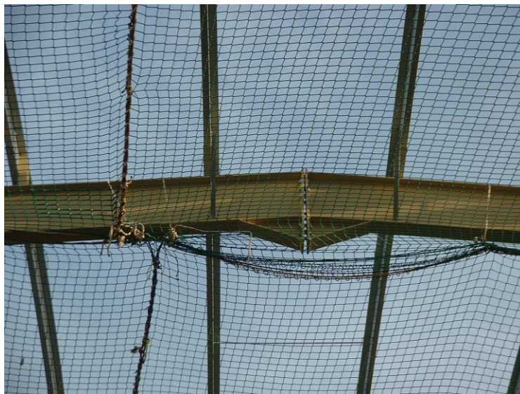
Image 2: Incomplete structural connections
