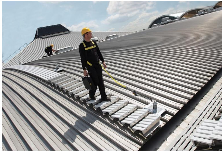
Latchways Constant Force fall protection and WalkSafe system on Kalzip standing seam roof. Image courtesy of Latchways plc
