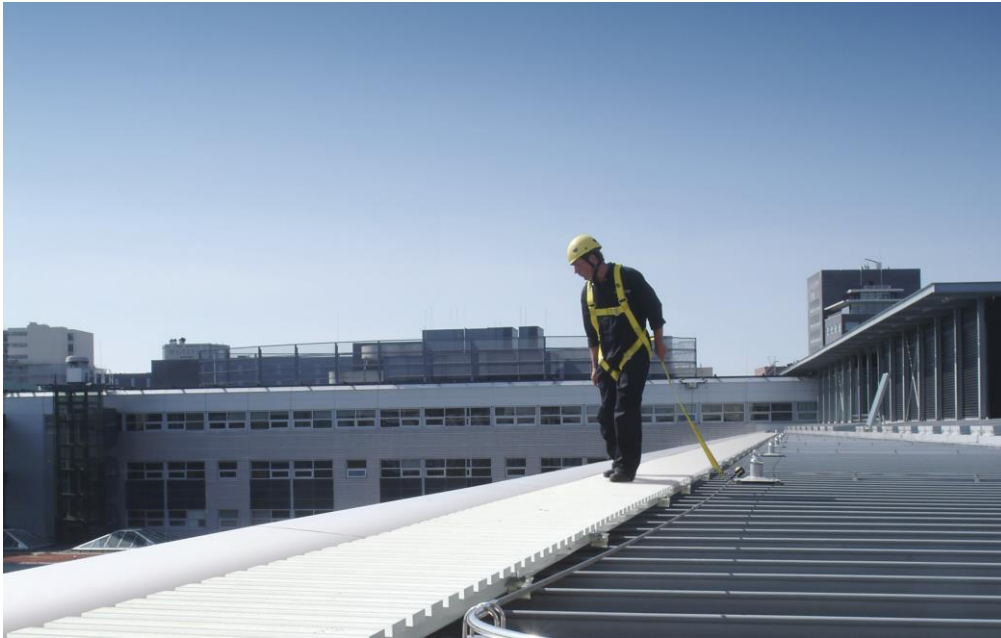
Collective fall protection of guardrail and walkway with accompanying cable system providing access to restricted areas. Image courtesy of Latchways plc
