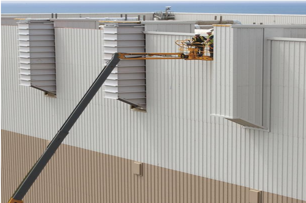
Trisomet 333 System insulated wall panels on the Pond Hall building at Sellafield. Photo courtesy of Tata Steel
